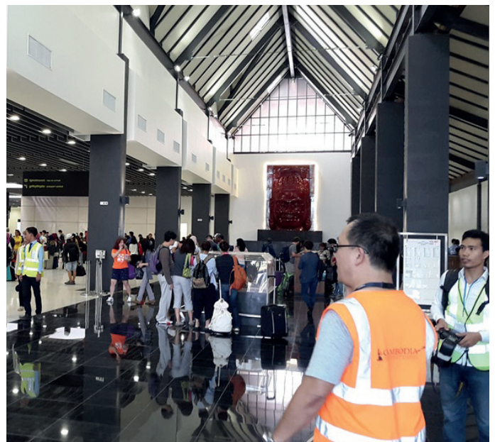
2. In Siem Reap, the handover of the new boarding area enabled the teams to begin renovating the spaces in the old terminal.
