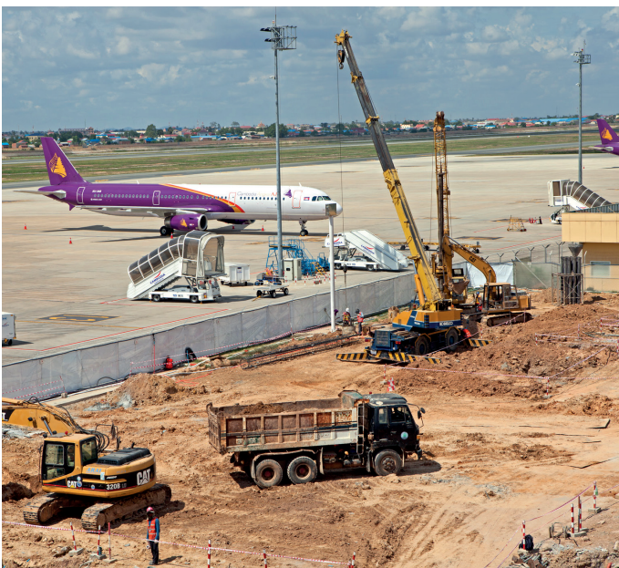
1. Bored pile construction at the foot of the runways in Phnom Penh.
