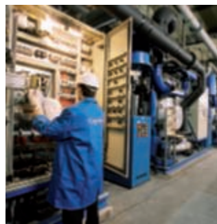
PUMPING STATION IN CHOISY-LE-ROI NEAR PARIS
