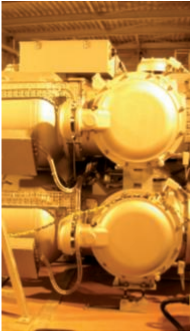
GIS SHIELDED STATION IN BELGIUM
